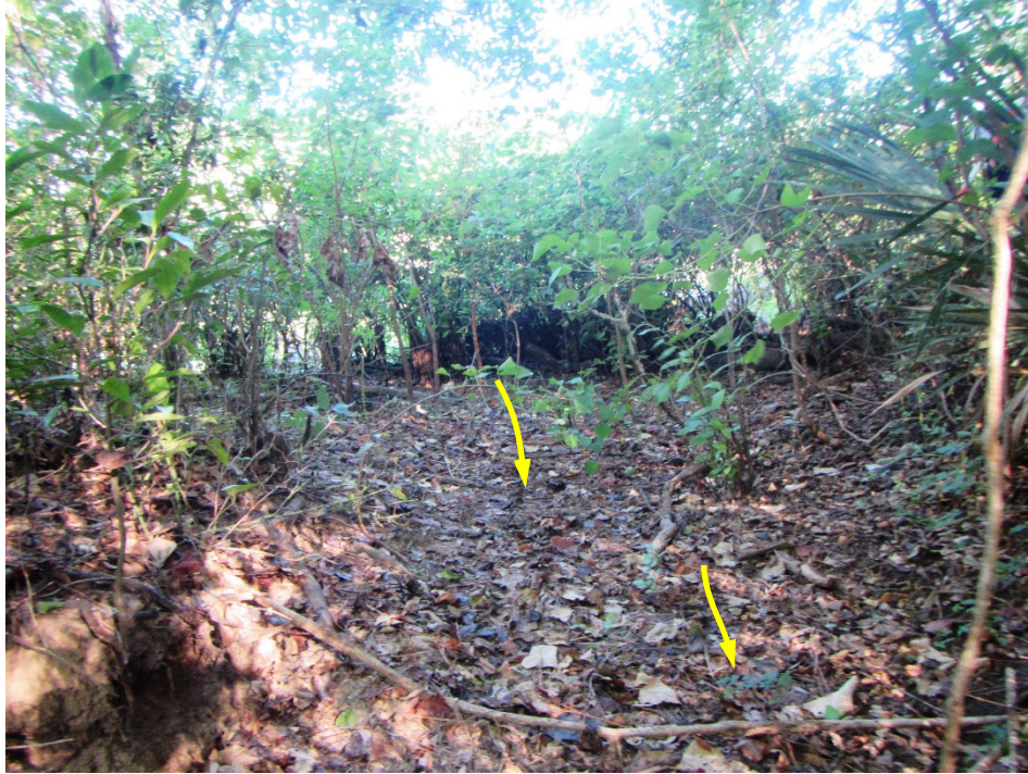
Photo 13. View of the spillway approach looking upstream. Note the dense brush and small tree growth obstructing the spillway approach. The direction of flow is noted by the arrows.
