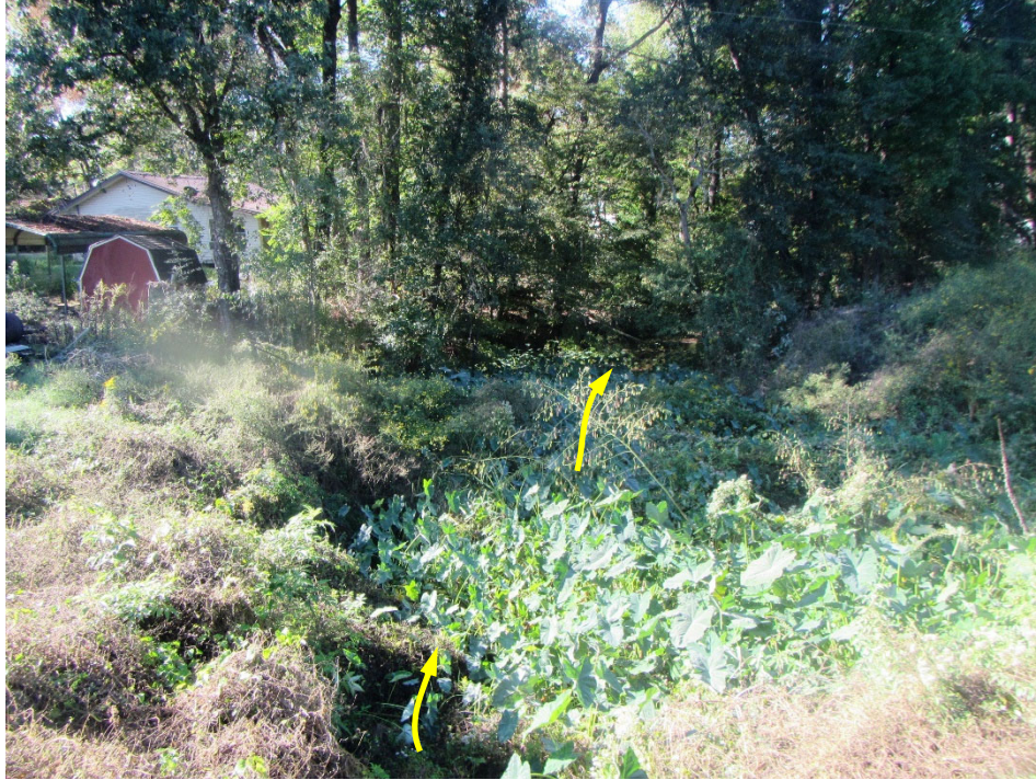
Photo 19. View of a downstream channel looking downstream from the roadway. Note the dense brush and tree growth along the channel and channel banks. The direction of flow is noted by the arrows.
