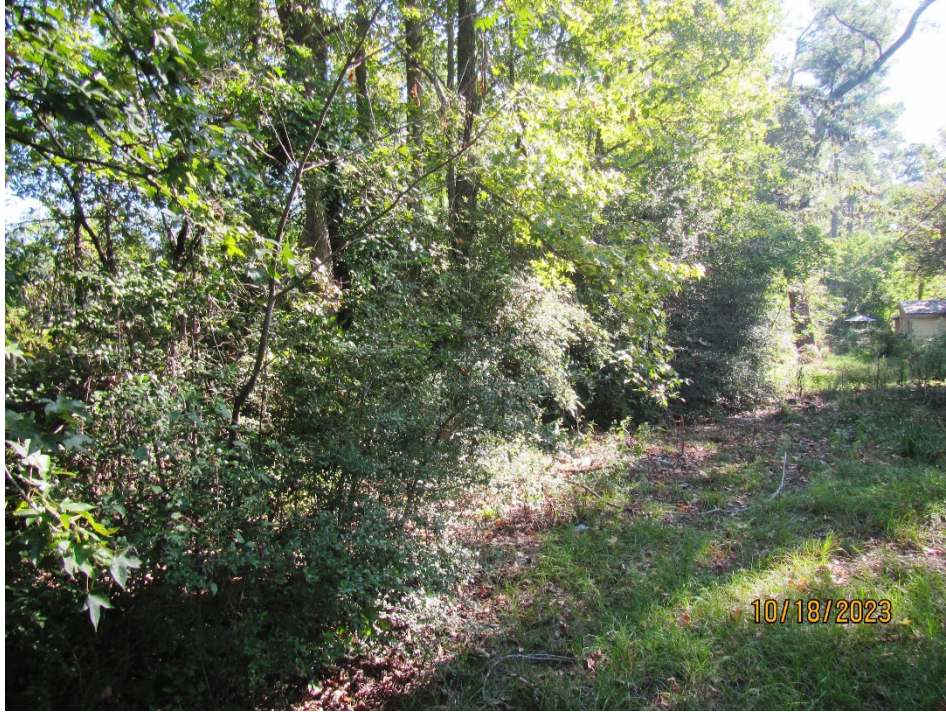
Photo 9. View of the densely overgrown brush and tree growth along the downstream slope looking left from the right end of the dam. Note the habitable residences along the downstream toe area.
