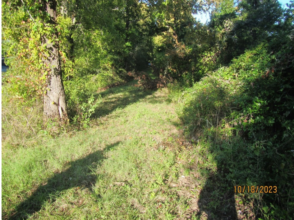
Photo 1. View of the crest looking right from the left end of the dam. Note the dense brush and tree growth along the slopes beginning to encroach the crest.
