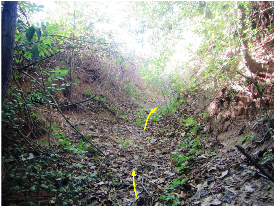
Photo 14. View of the spillway channel looking downstream. Note the vegetative growth along the channel banks encroaching on the spillway channel. The direction of flow is noted by the arrows.
