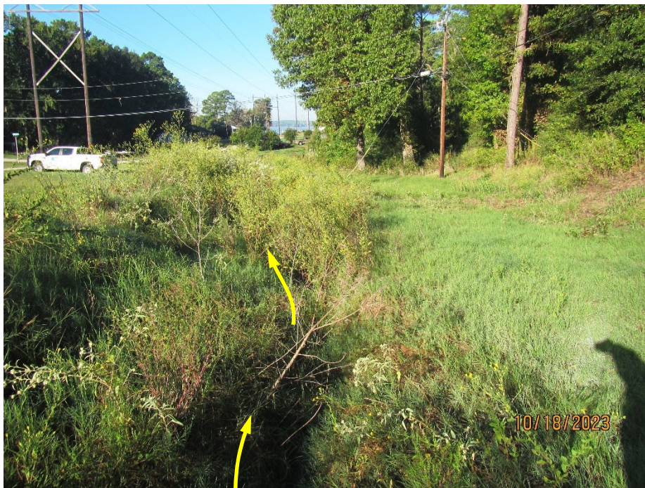
Photo 16. View of the shallower section of the spillway channel (approximately 2-feet deep) looking downstream. The direction of flow is noted by the arrows.
