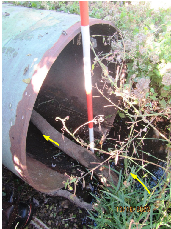
Photo 18. View of the 3-foot diameter steel culvert under East High Line Road. The culvert was obstructed with some dry wood debris and just engaged with flow from the downstream pond. The direction of flow is noted by the arrows.
