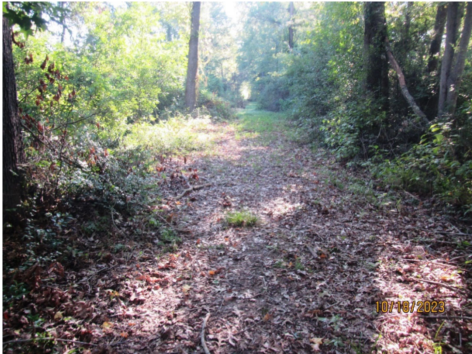
Photo 2. View of the crest looking left from the right end of the dam. Note the brush and tree growth along the slopes and the lack of grass cover along the crest.
