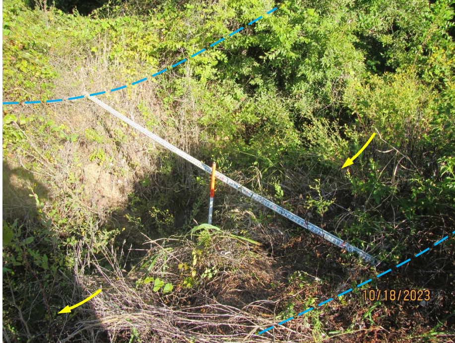
Photo 15. View of the obscured spillway channel (estimated dashed lines) looking upstream. The dimensions of the spillway channel were approximately 15-feet wide and 6-feet deep at this section of the channel with encroaching brush vegetative growth. The direction of flow is noted by the arrows.
