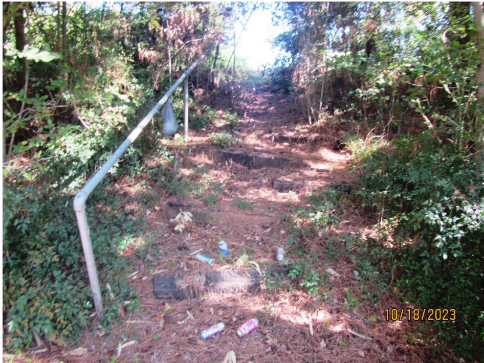
Photo 12. View of a staired foot path and handrail along the downstream slope near the mid-right end of the dam. Note the railroad ties used as steps along the slope.
