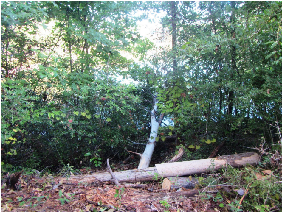
Photo 6. View of a downed tree along the crest/upstream slopes edge, near the mid-right side of the dam.
