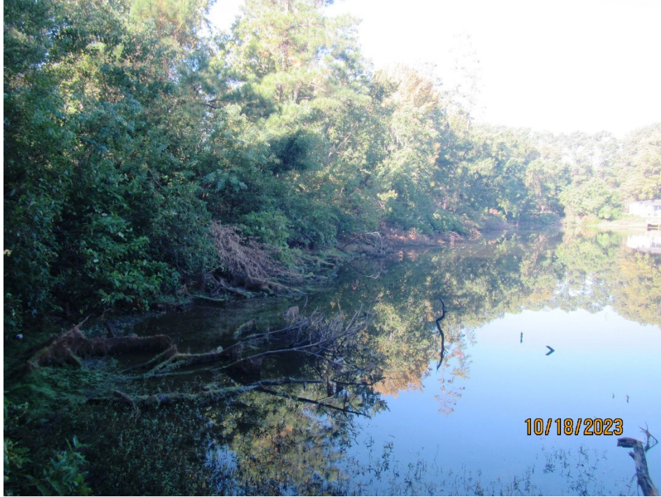
Photo 3. View of the upstream slope looking right from the left end of the dam. Note the dense brush and tree growth along the length of the slope.
