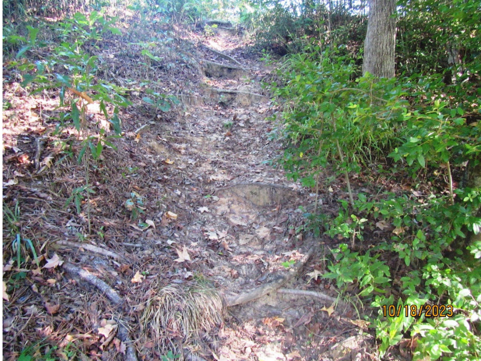
Photo 11. View of a trail observed on the downstream slope near the middle of the dam. Note the exposed tree roots crossing the trail as a result of runoff erosion.
