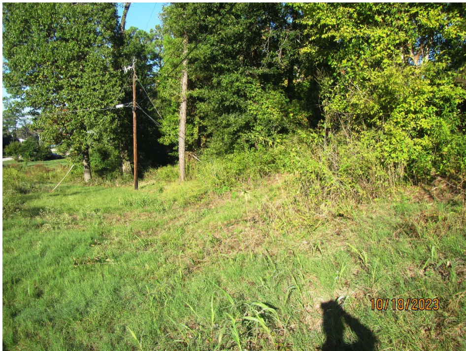
Photo 8. View of the densely overgrown brush and tree growth along downstream slope looking right from the left end of the dam. Note the utility lines traverse across the length of the downstream toe area.
