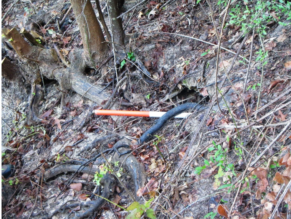
Photo 7. View of a burrow along the upstream slope, about 2-feet deep, near the middle of the dam.
